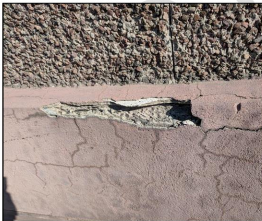
Photo 7: Debonded parging on the south elevation [JCAL 2018].
