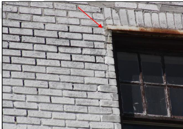
Photo 6: Third floor window on east elevation with deteriorated bricks around the perimeter [JCAL 2018].
