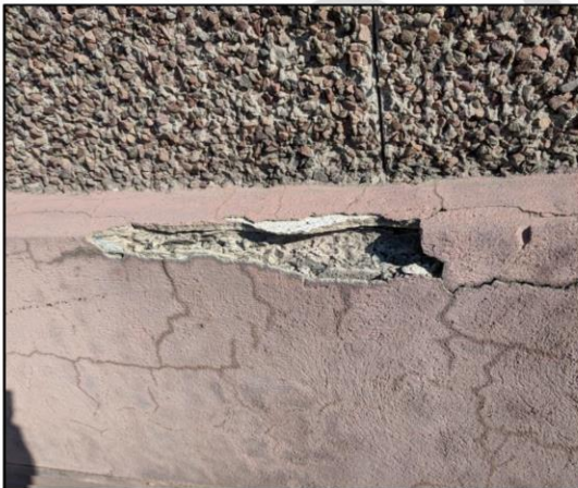
Photo 7: Debonded parging on the south elevation [JCAL 2018].
