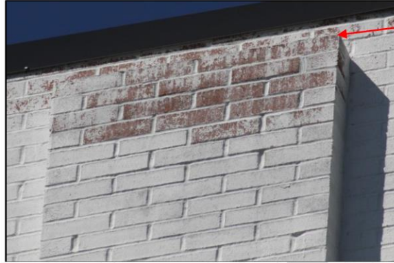
Photo 9: Top of pilaster, on east elevation, with no cap flashing [JCAL 2018].
