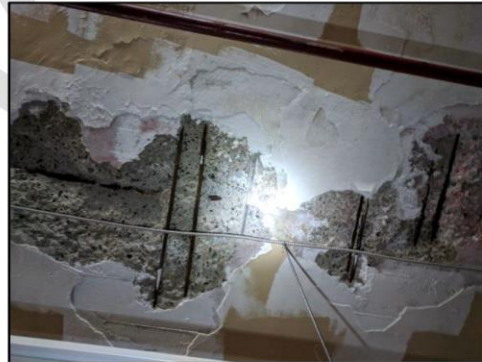
Photo 3: Corroding rebars have caused the concrete to spall on the underside of the third floor. [JCAL]
