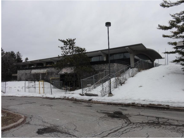
Photo 7 – View of West Annex (under demolition) on the northern portion of Parcel C, looking east.
