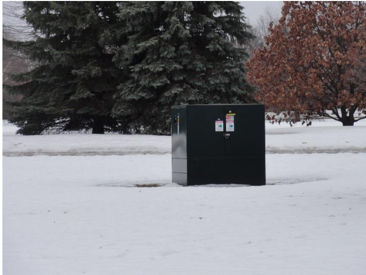
Photo 11 – View of a typical concrete pad-mounted transformer located west of West Annex Building; however, snow cover restricted inspection of ground conditions in the vicinity of this PCA.
