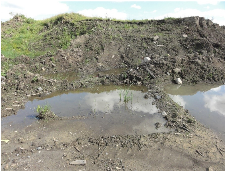
Photo 6 – Stockpiles of stripped topsoil from the Site on the southern portion of the Site, looking southeast.
