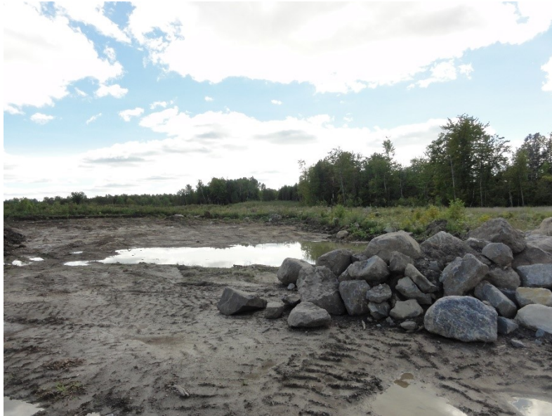
Photo 3 – View of southern portion of the Site with topsoil stripped off, looking southwest.
