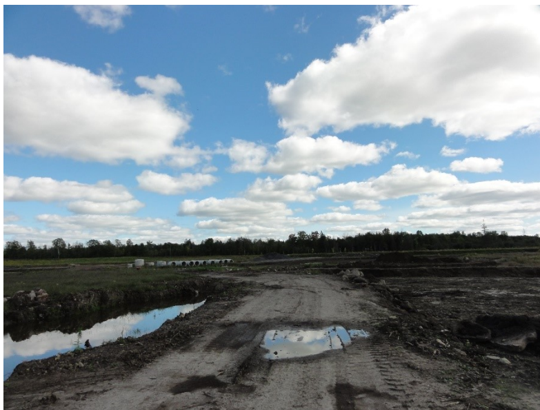
Photo 4 – View of construction road providing access to the Site from southeast corner of the Site, looking southeast.
