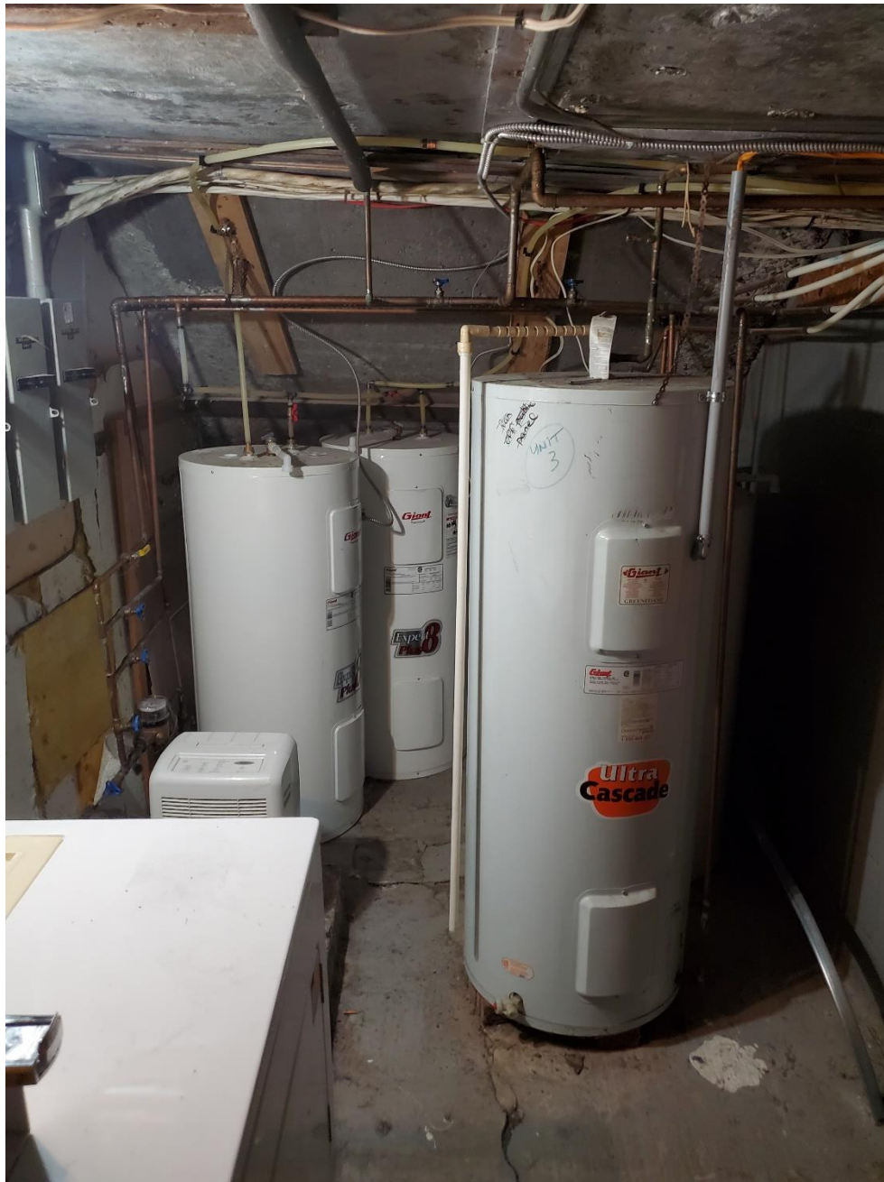
Photo 2: Facing east, hot water tanks located in the basement. The site is service by municipal water.
