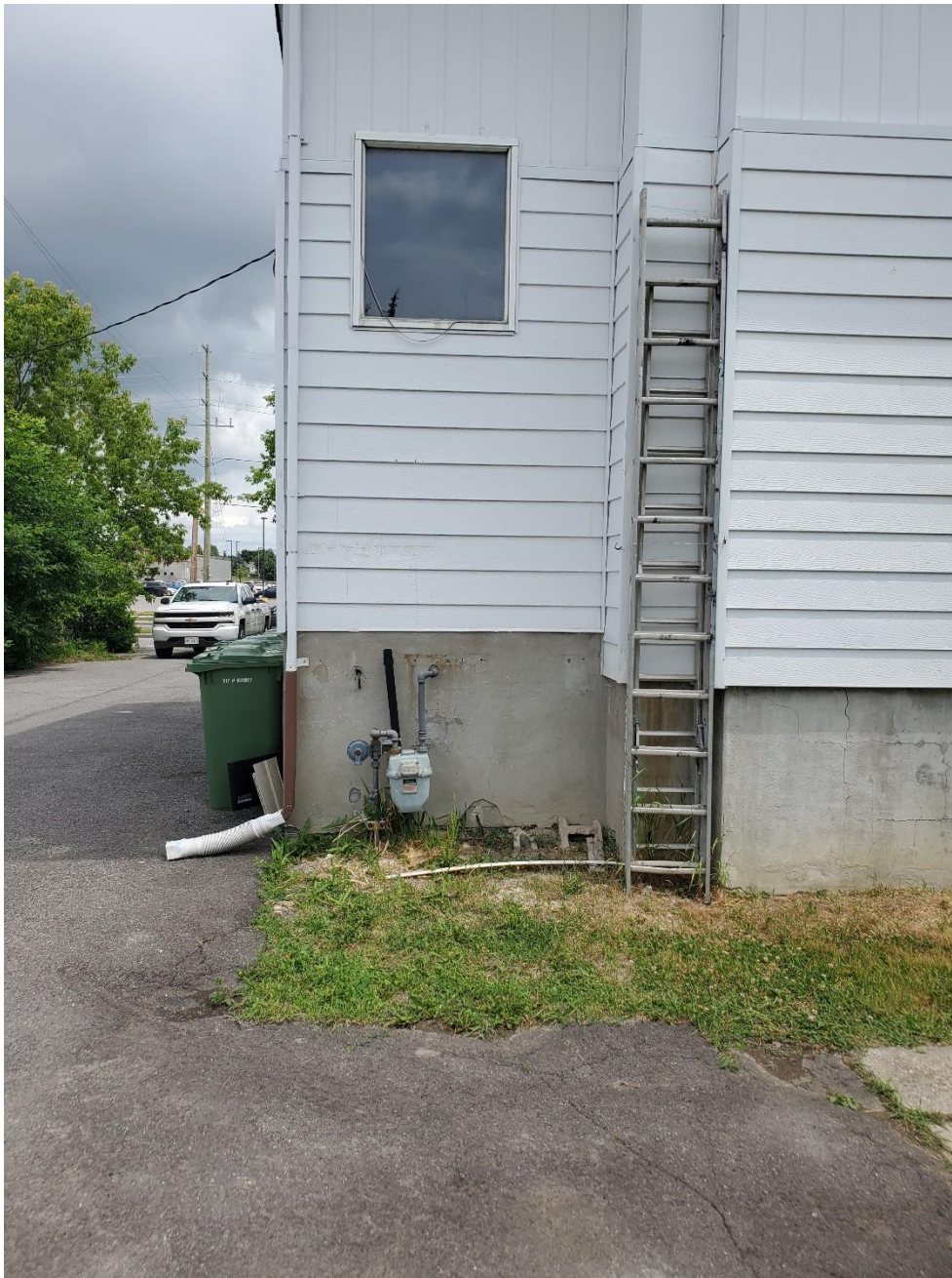
Photo 4: Facing east, gas enters the property from the west side of the building.
