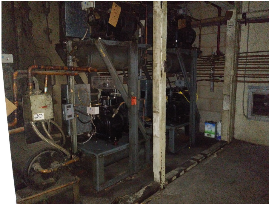
Photograph 10: View of the refrigeration equipment in the penthouse level of the former grocery store in the northwest portion of the north commercial plaza building.
