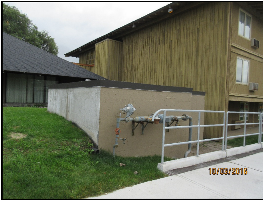
Photograph 9: Photograph illustrates southernmost access to the basement level, situated along Meath Street, facing east-southeast.
