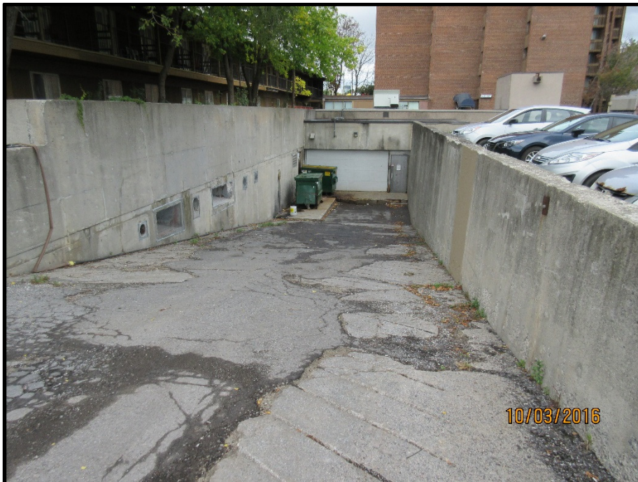
Photograph 6: Photo illustrates the access ramp to the shipping and receiving area, south of the former Centennial Ballroom, facing north.
