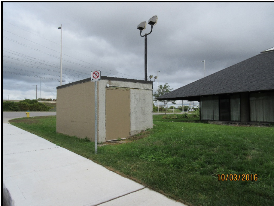
Photograph 10: Photograph illustrates northwest corner of Phase I Property and exterior access to basement of the Beachcomber (former nightclub), facing northeast.
