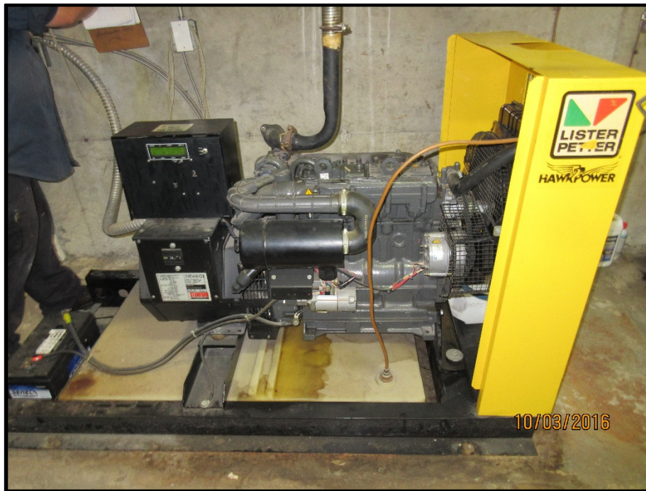
Photograph 11: Photograph illustrates diesel generator in the Beachcomber mechanical room.
