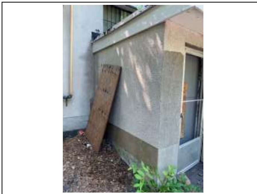
Photograph 36: View of suspected asbestos-containing pebble dash exterior finish on the north façade of the building.
