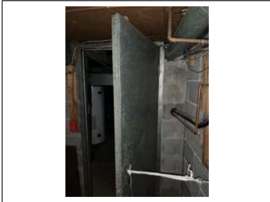
Photograph 15: View of fire resistant door in the basement furnace room with a suspected asbestos-containing interior liner.
