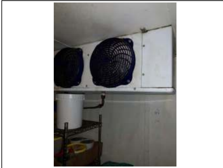
Photograph 29: View of the inside of the walk-in refrigerator in the kitchen.
