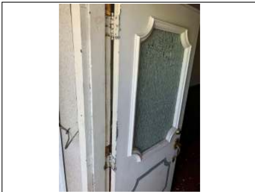
Photograph 8: View of the roof access entrance to the second floor apartment unit.
