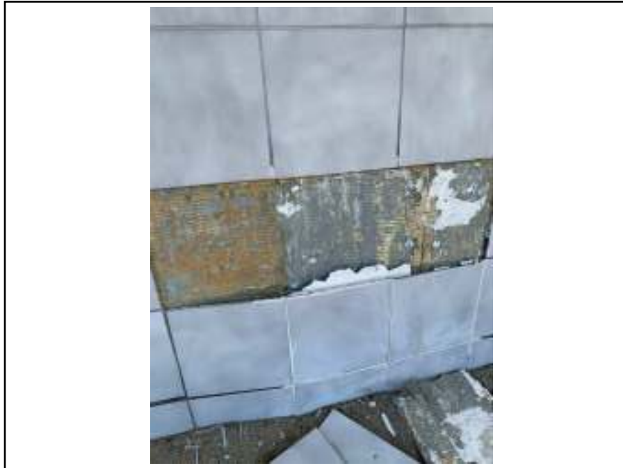
Photograph 39: View of suspected asbestos-containing grout behind exterior ceramic tile along the south, west and east facades of the building.
