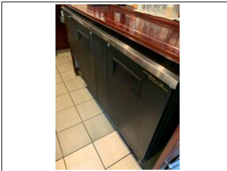
Photograph 32: View of the drink cooler in the bar area, potentially ODS containing.
