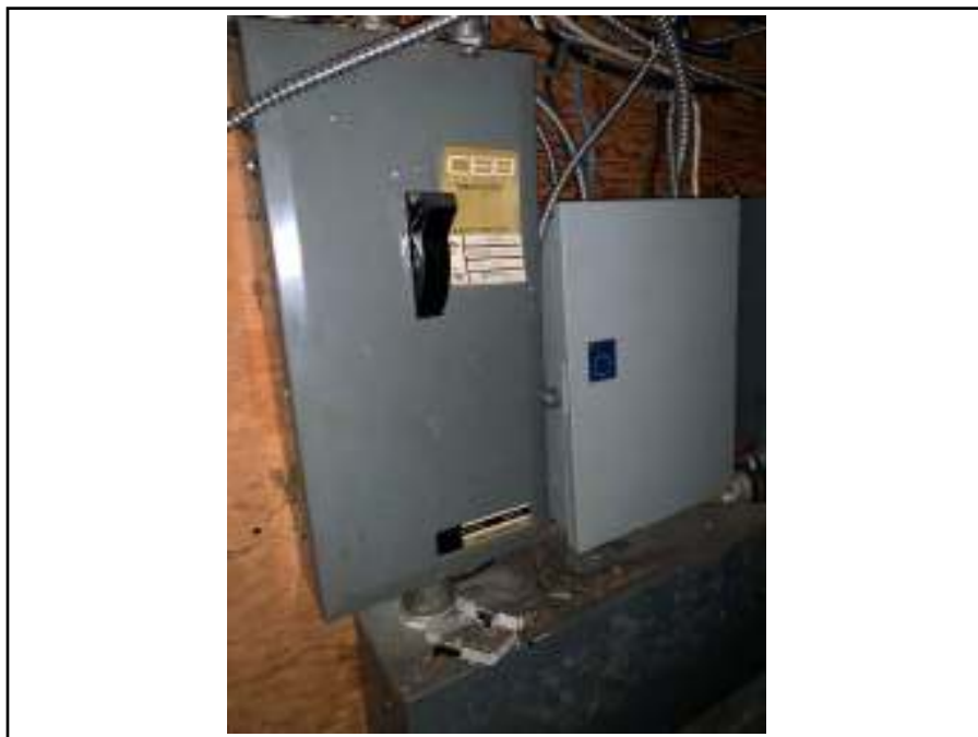
Photograph 16: : View of the electrical panel along the south wall of the basement.
