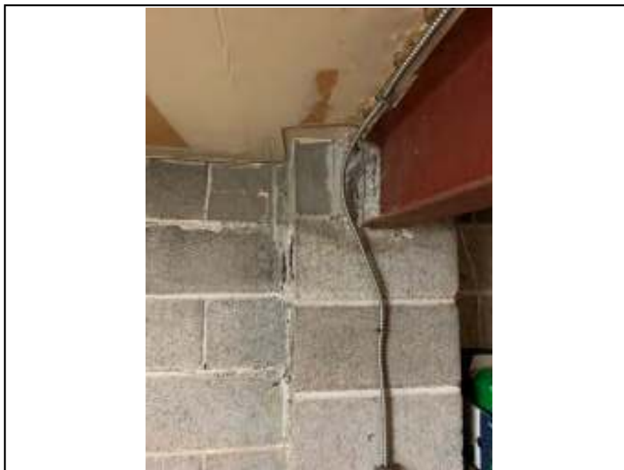
Photograph 14: View of suspected asbestos-containing wall parging associated with ceiling beams in the basement.
