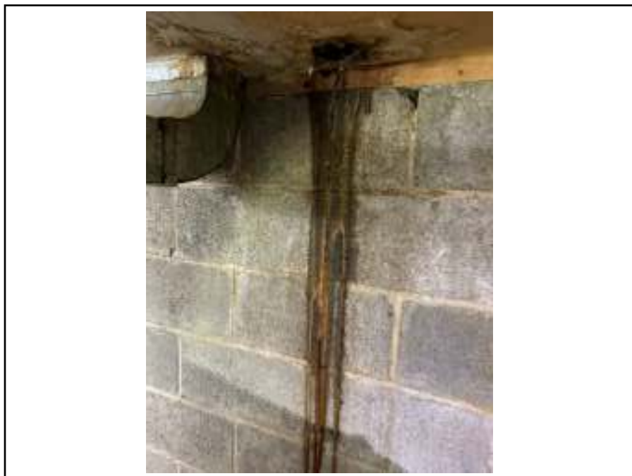
Photograph 12: View of grease staining on basement walls.
