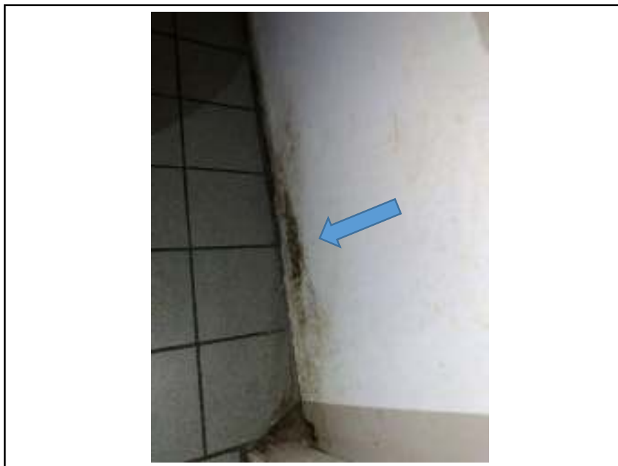
Photograph 28: View of suspected mould growth along the baseboards of the main floor washroom in the kitchen area.
