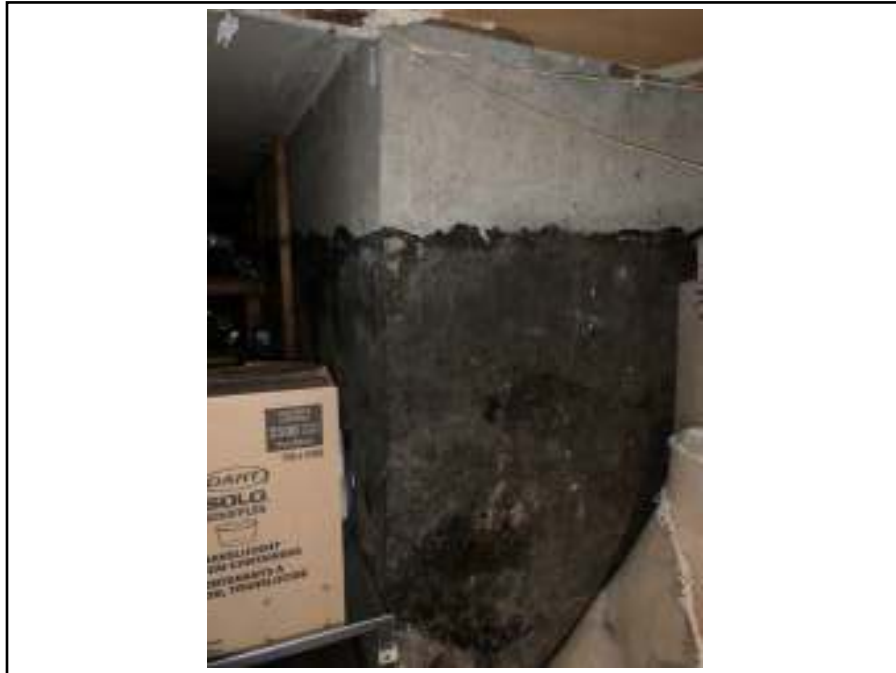
Photograph 9: View of suspected asbestos containing wall parging in the basement.
