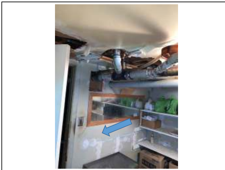
Photograph 24: View of suspected asbestos-containing drywall joint compound in the basement.
