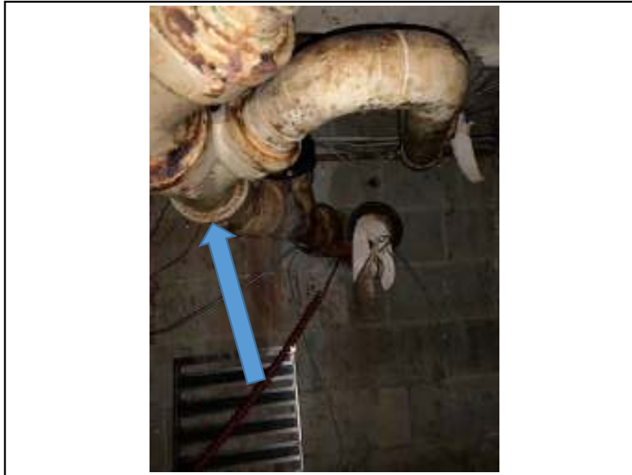
Photograph 19: View of cast iron drain along the south wall of the basement and suspected asbestos-containing oakum joint packing.
