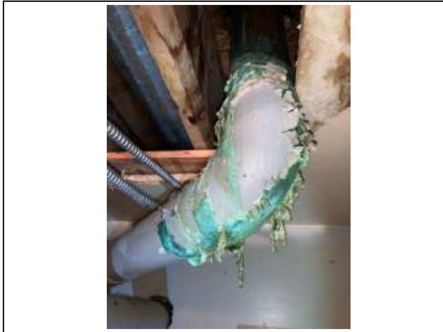
Photograph 25: View of suspected lead-based paint on drainage pipes in the basement.
