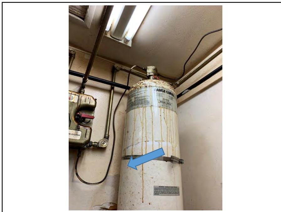
Photograph 26: View of wet chemical fire suppression system in the kitchen.
