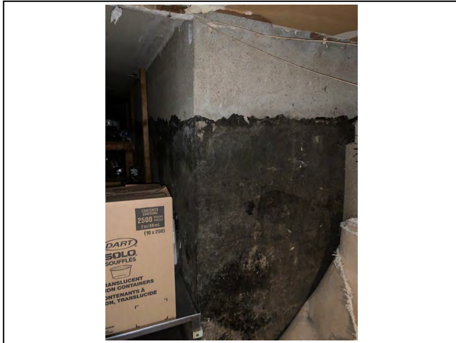
Photograph 9: View of suspected asbestos containing wall paring in the basement.
