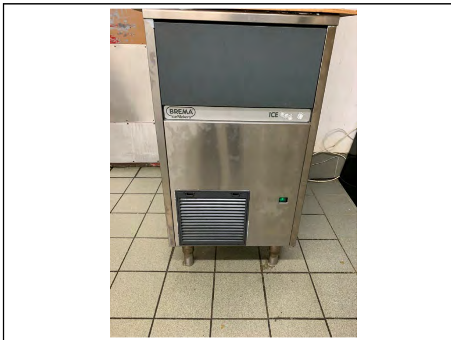
Photograph 30: View icemaker in the kitchen, potentially ODS containing.
