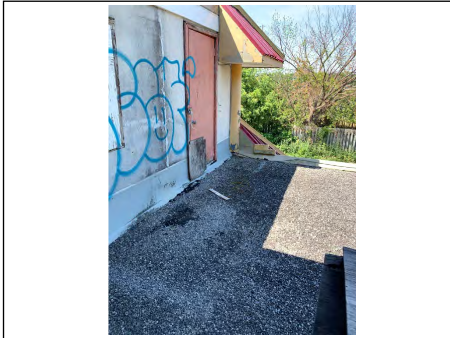
Photograph 33: View of the roof and exterior wall of the second floor apartment unit.
