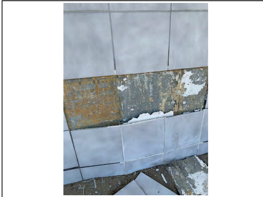
Photograph 39: View of suspected asbestos-containing grout behind exterior ceramic tile along the south, west and east facades of the building.
