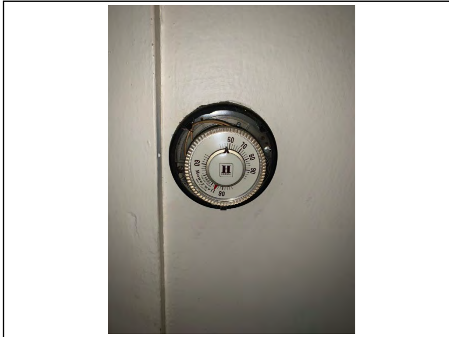
Photograph 35: View of suspected mercury-containing thermostat in the second floor apartment unit.
