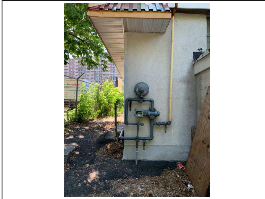
Photograph 37: View of gas line point of entry on the north east corner of the building.
