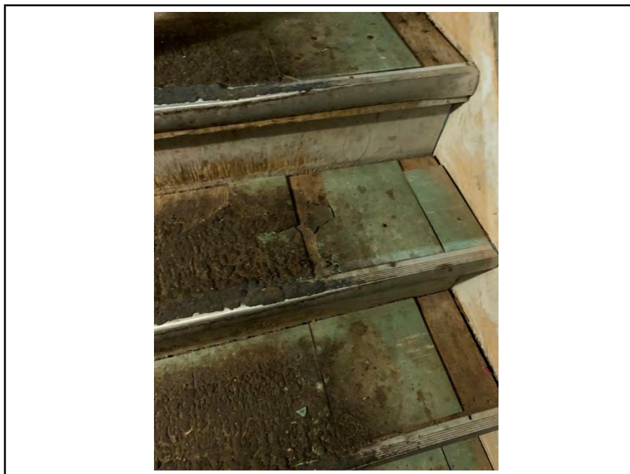
Photograph 22: View of suspected asbestos-containing 9'X9' Vinyl Floor Tile in the basement stairwell.
