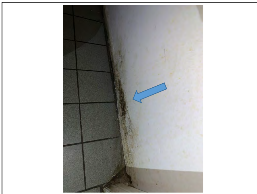
Photograph 28: View of suspected mould growth along the baseboards of the main floor washroom in the kitchen area.
