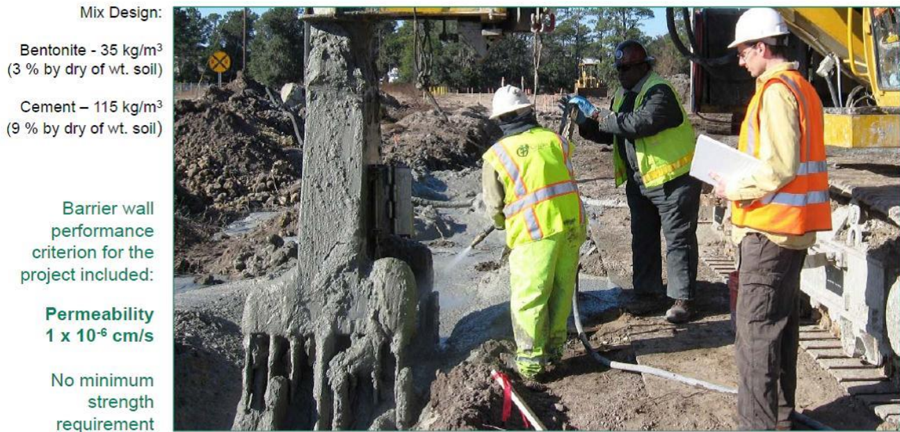
Figure 5.7 Outer Barrier Wall Construction using Cutter Soil Mixing at US EPA's Brunswick, Georgia Superfund Site
