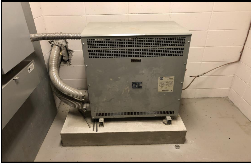
Photograph 5: View of a dry-type, pad-mounted transformer, located within the ground floor electrical room.
