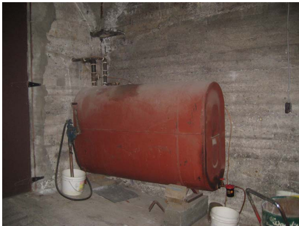
Photograph 16: View of the diesel AST located in the former coal storage room and used to fuel the backup generator.
