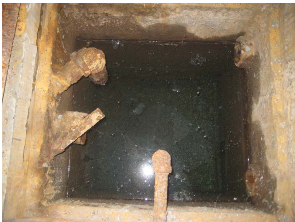
Photograph 18: View of the water in the sump located in the boiler room.
