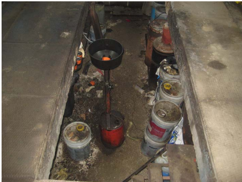
Photograph 23: View of the maintenance pit located in the garage, the staining on the concrete floor and the oils/lubricants stored in containers in the pit.
