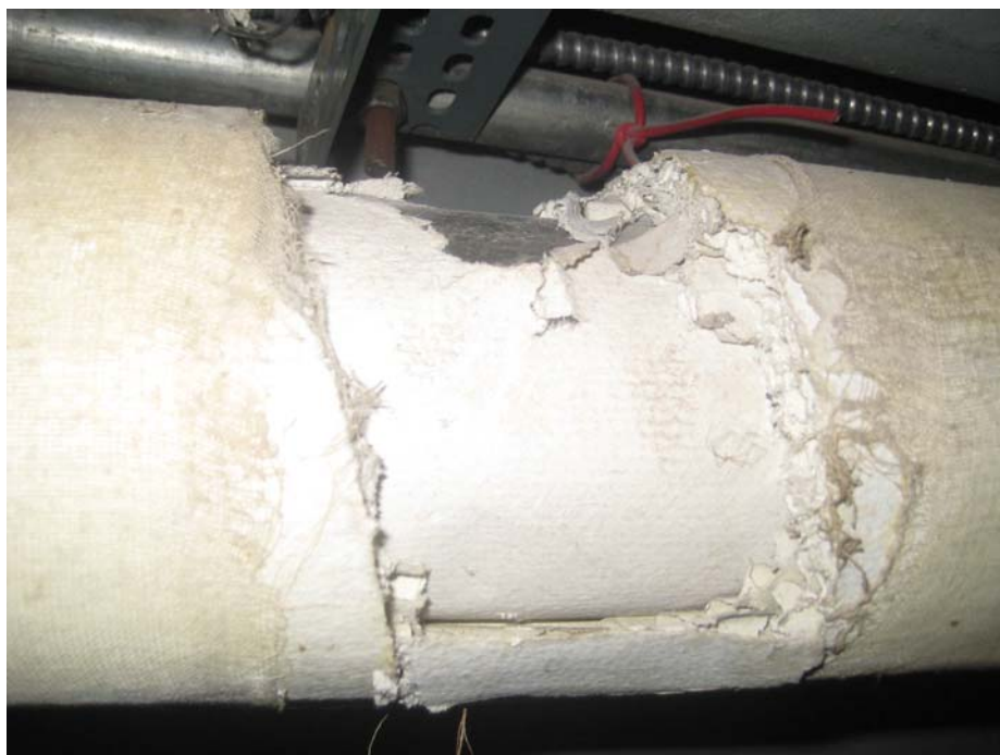
Photograph 24: View of the potential ACMs in the form of parging cement insulation on piping in the boiler room.
