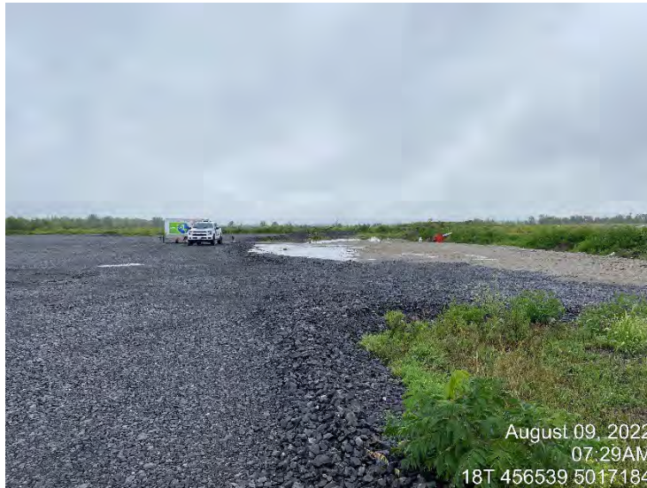
Photo 1 - View of drilled water well on the Site used during pumping test and proposed building area showing ground improvement.
