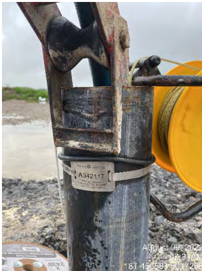
Photo 3 - Wellhead at pumped water well A342117.
