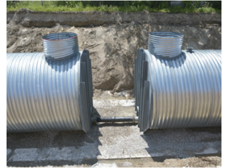
GALVANIZED CSP FIREWATER TANK SYSTEM
