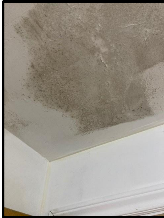
Photograph 3: Mold growth in the basement of 257-259 King Edward Avenue.
