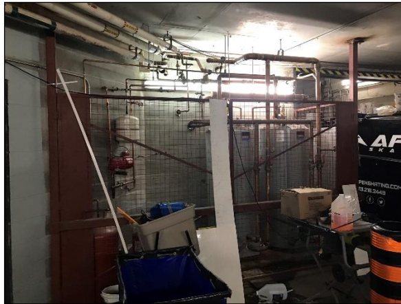
Hot water holding tanks
