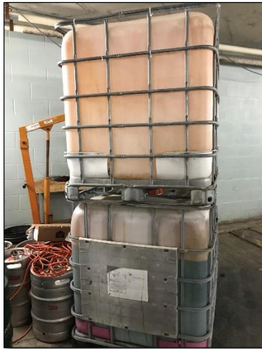
Brine storage from rink cooling pad
