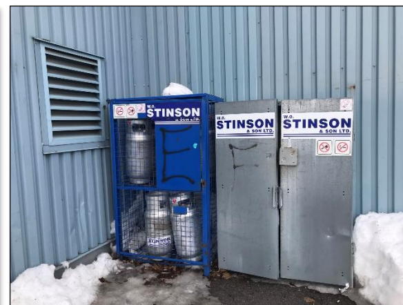
Propane canister storage
