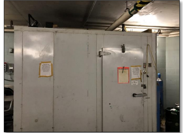
Lower floor - commercial refrigeration unit
