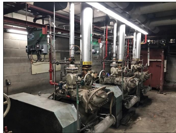
Plant room – brine pumps
