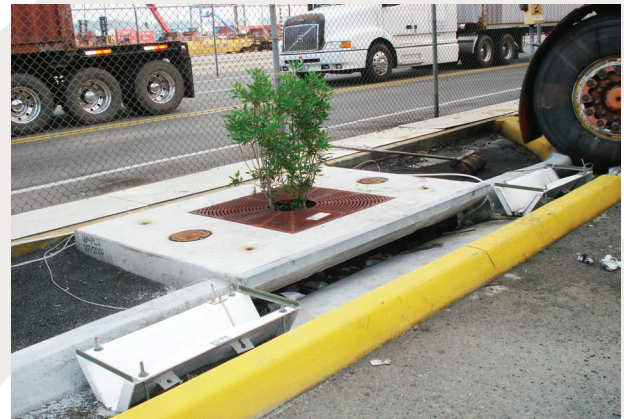
Filterra™ monitoring unit at a port.
