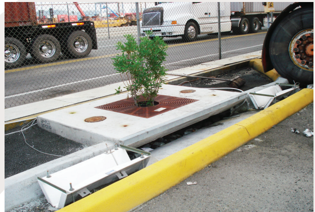
Filterra™ monitoring unit at a port.
