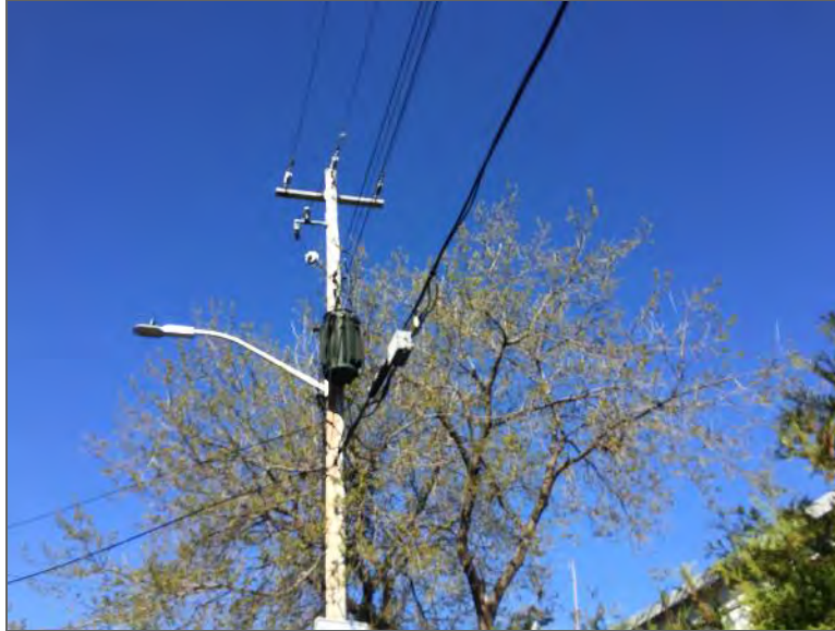
Photo 9 – PCA #2 Transformer observed on the south portion of the Phase One Property.
