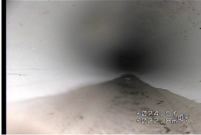
Figure#19: A view to the 0% water level and material change to PVC at 22.8 meters from the top of (CB1).
