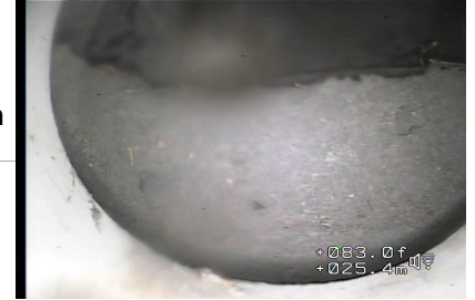
Figure#20: A view to the end point CB1 and flow restrictor at 25.4 meters from the top of CATCH BASIN 1 (CB1).
