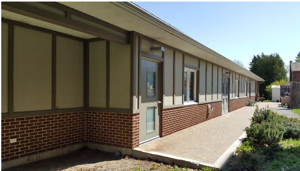
Photo 6 - View of the meeting hall building on the north portion of the Site; view is looking east.
