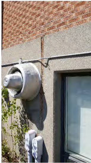
Photo 10 - View of former location of suspected exterior vent and fill pipes on the east Side of the Church building.
