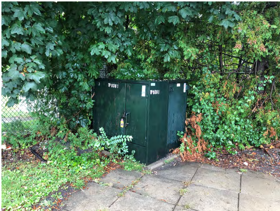
Photo 8 Photo showing the pad-mounted transformer in the central portion of the Site
