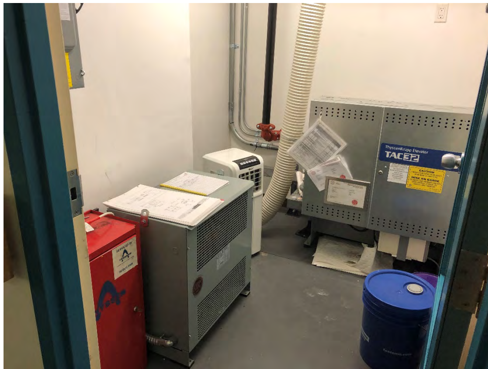
Photo 22 Photo showing the elevator maintenance room at Ellwood House Seniors' Residence
