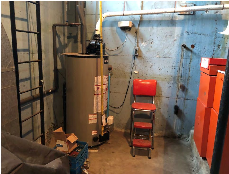
Photo 11 View of the historic fuel oil AST location and former fill pipes on the church mechanical room
