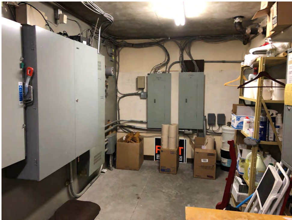
Photo 20 View of the electrical room in Ellwood House Seniors' Residence
