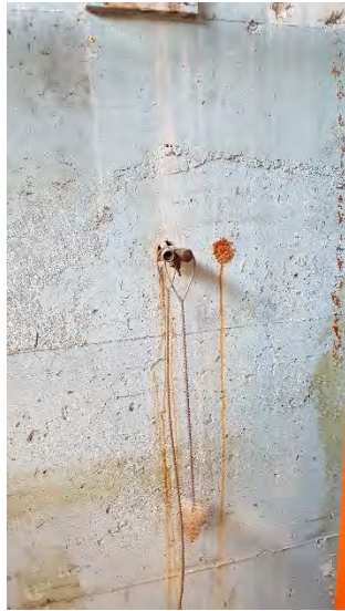
Photo 9 - View of former/disconnected suspected vent and fill pipes on the interior of the mechanical room of the Church building. The piping is suspected to have been associated with a historical interior aboveground storage tank.
