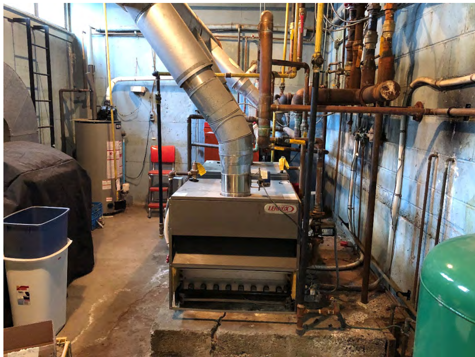
Photo 10 Photo showing the mechanical room in the basement of the church
