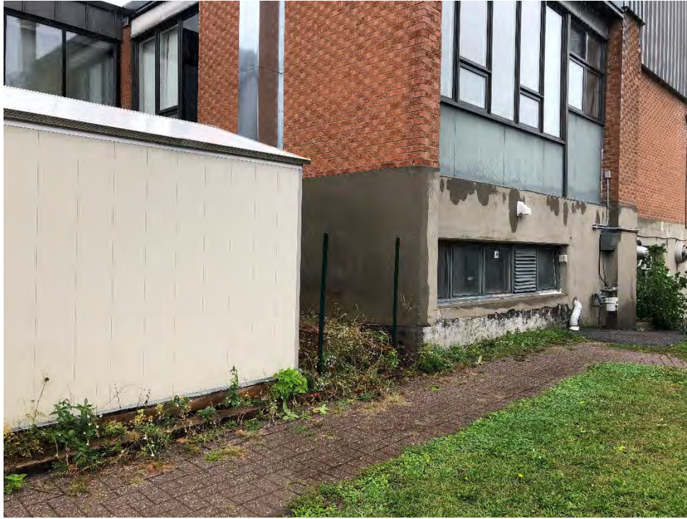
Photo 9 Photo showing the location of the location of the historic fuel oil tank fill pipes on the east side of the church
