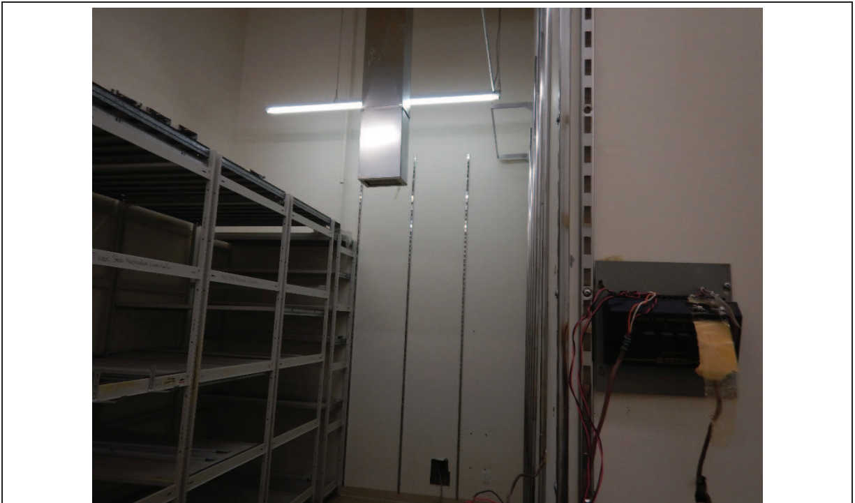
Photo 8: Typical electrical service in the vacant commercial retail space on the Phase One Property - 2021
