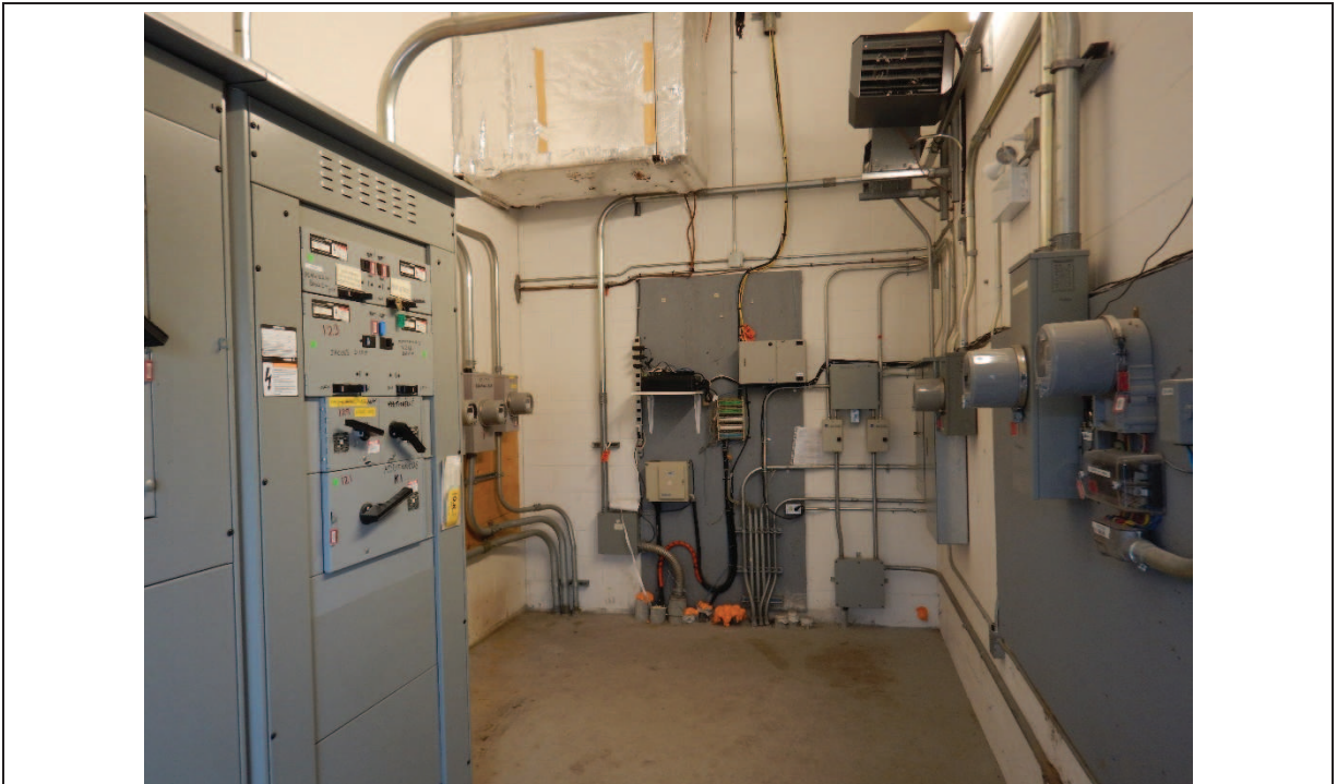
Photo 10: Transformer room for the vacant commercial retail space and Cineplex on the Phase One Property - 2021
