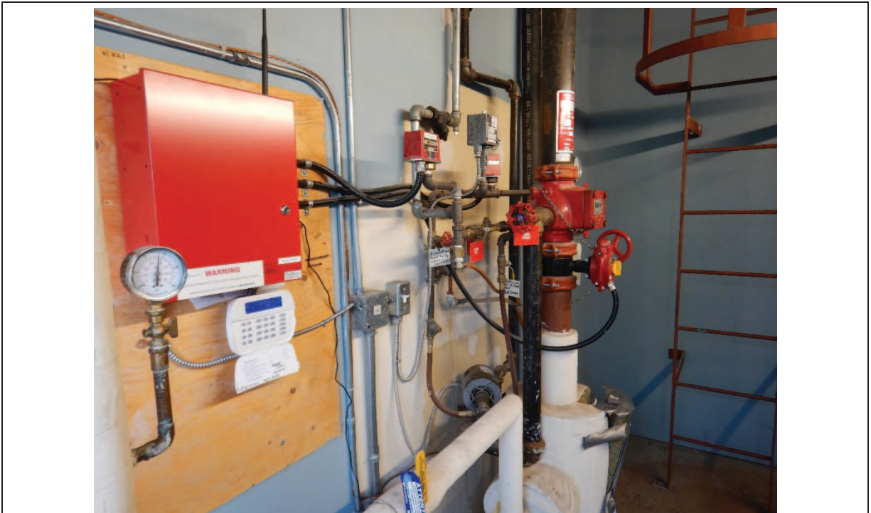
Photo 9: Water service in the vacant commercial retail space on the Phase One Property - 2021
