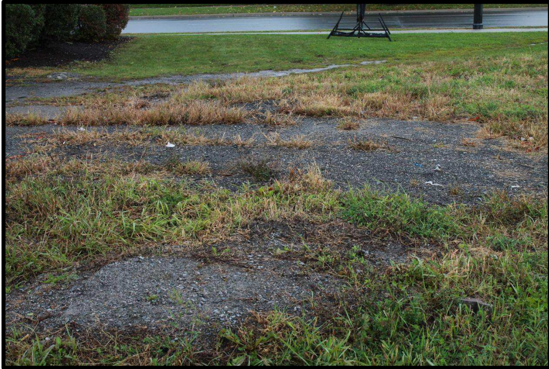
Figure 5. Asphalt adjacent to Watters road (D004)
