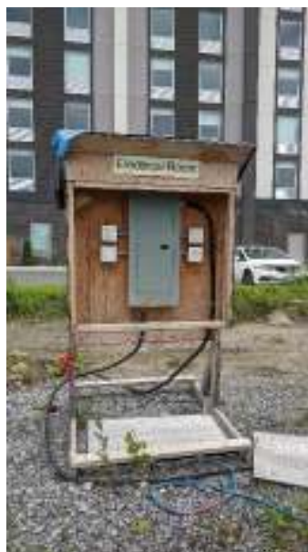
Photograph 10: On-site electrical service located on northeast corner of property adjacent to mobile office trailer.
