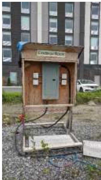
Photograph 10: On-site electrical service located on northeast corner of property adjacent to mobile office trailer.
