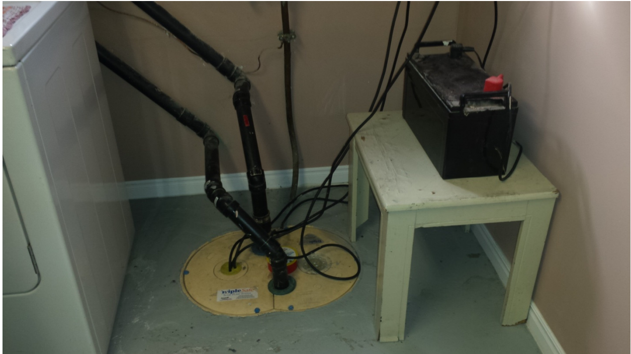
Photograph 3: Sump pit (with two submersible pumps) and backup battery in the basement of 3996 Innes Road.
