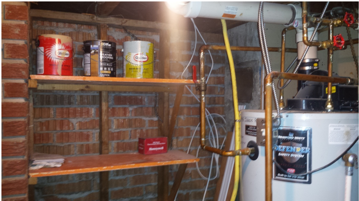
Photograph 4: View of the basement boiler room (3996 Innes Road). The brick wall is part of the sealed chimney.
