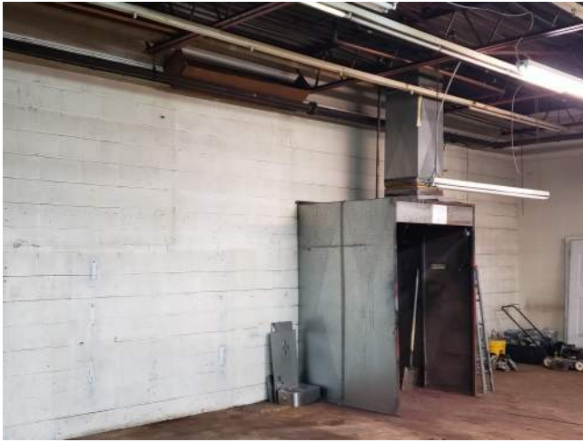
Photo 7: View of former spray booth located on the western wall in the northern portion of the Site building.
