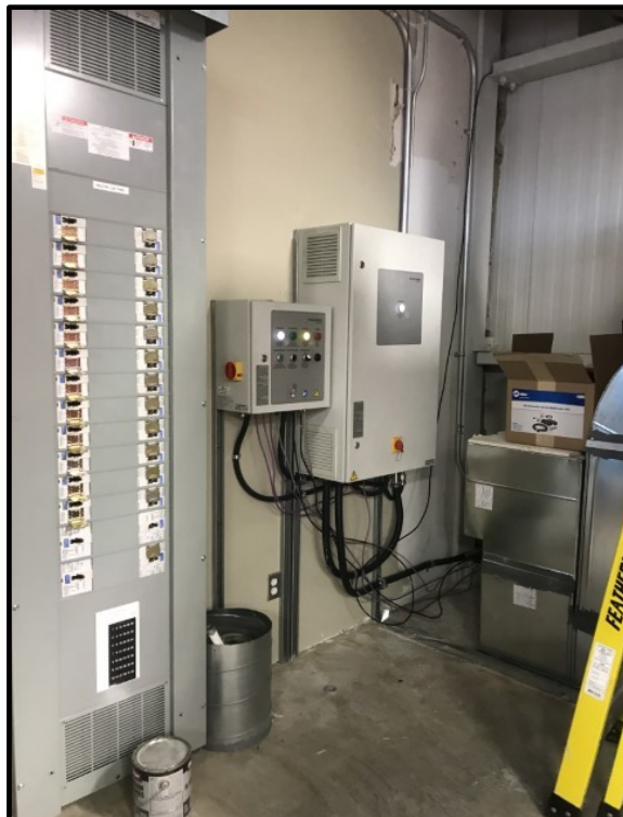
Photo 18: Electrical unit in welding training area.
