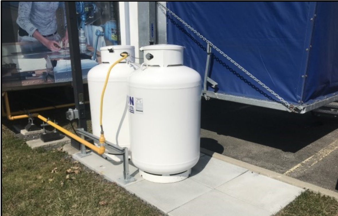
Photo 31: Photo of propane cylinders stored vertically on a concrete pad, to the south of the Site property.
