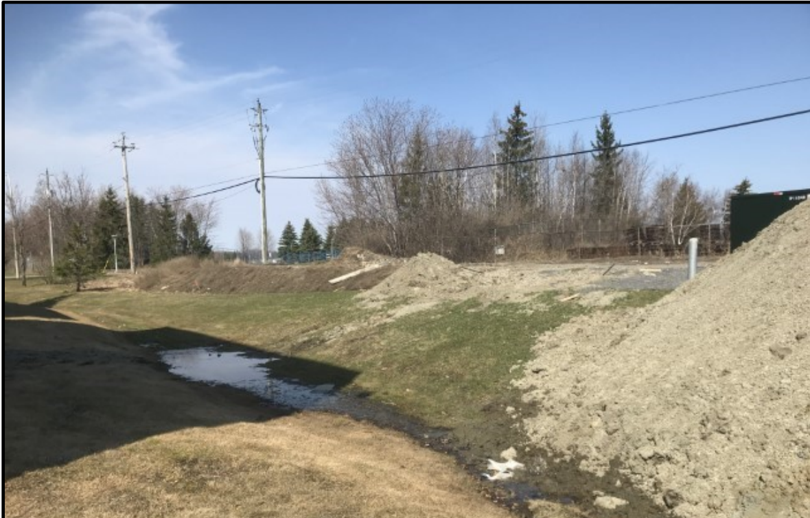
Photo 23: West-facing view of the drainage ditch, native stockpiles, and north boundary of the Site.
