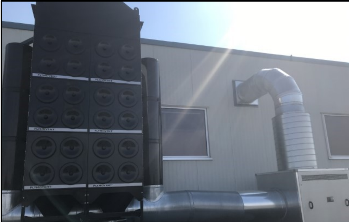
Photo 19: Central extraction fan with two drums for the collection of welding dust.
