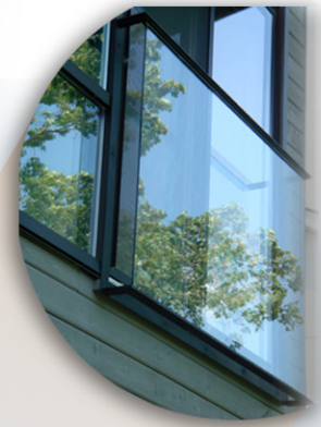
MODERN JULIET BALCONIES - Anodised Aluminum Handrails, With Satin Black Finish To Match D/W Frames & Tinted Grey Glass Panels
