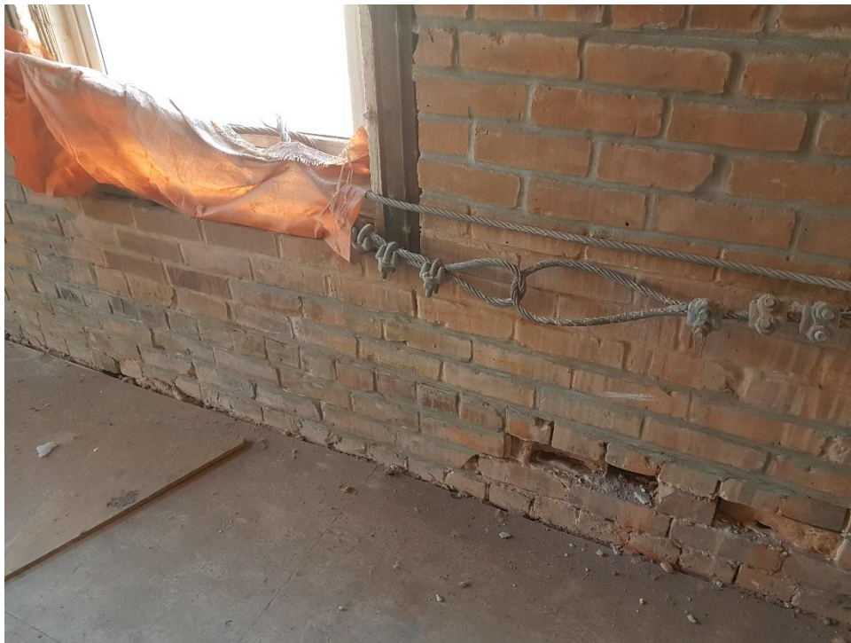
Photograph 10: Area of noted brick deterioration on the interior wythe of second floor, north wall.
