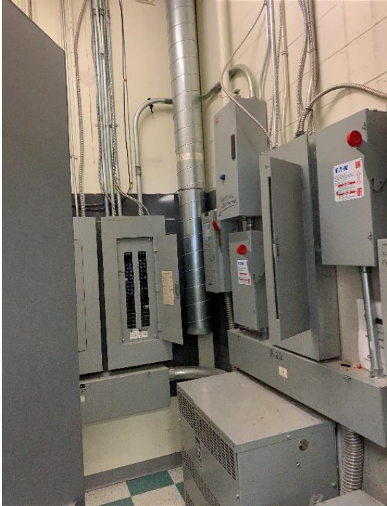
Photo 1: Power Room Located at the Site (Inside the Building)
