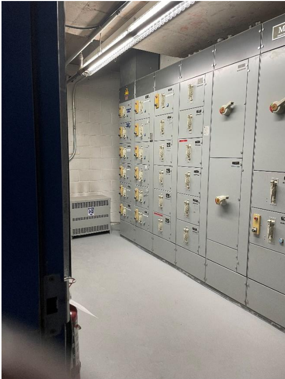
Photo 7: Electrical/Telephone Room in Parking Garage P1 (Phase One Property)
