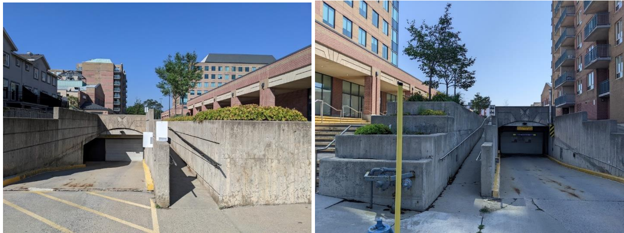
Photo 3: View of existing underground parking access to development site. Left: facing west. Right: facing east.
