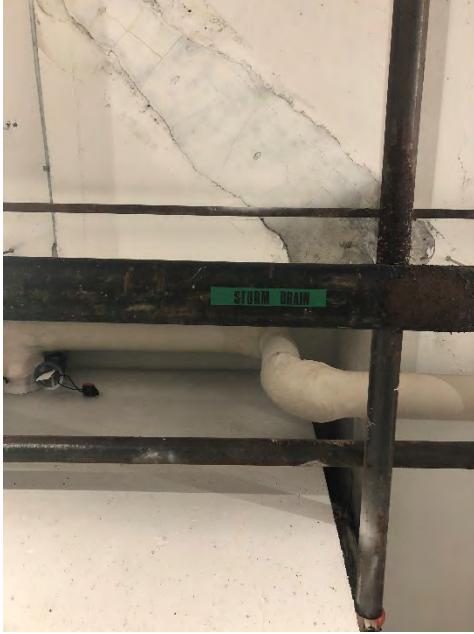
Photo 21 – Interior of mechanical room, second sub-level parking
