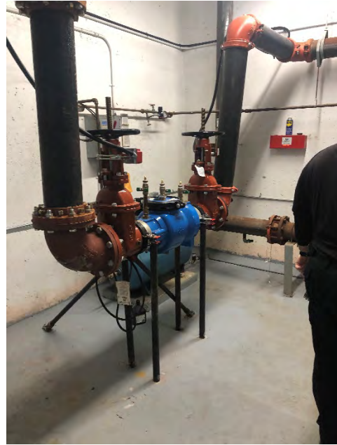
Photo 18 – Mechanical room interior, second sub-level parking
