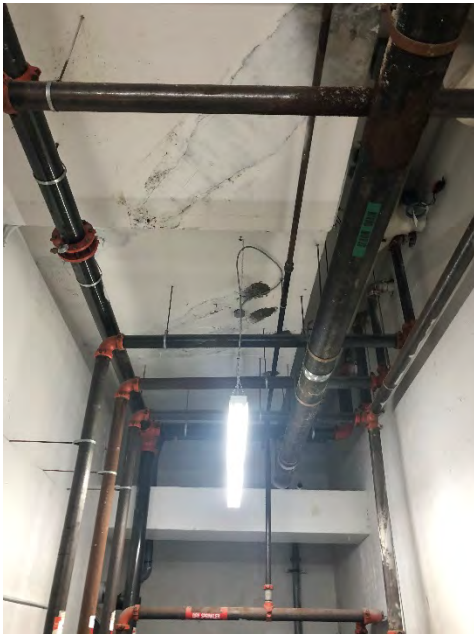
Photo 19 – Ceiling of mechanical room, second sub-level parking
