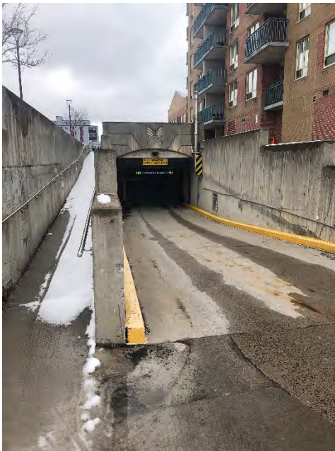
Photo 3 – Western entrance to the Holland Cross underground parking garage coming from Holland Avenue, looking east
