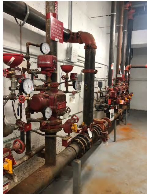
Photo 20 – Interior of mechanical room, second sub-level parking
