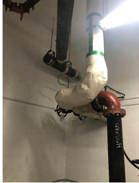
Photo 22 – Interior of mechanical room, second sub-level parking
