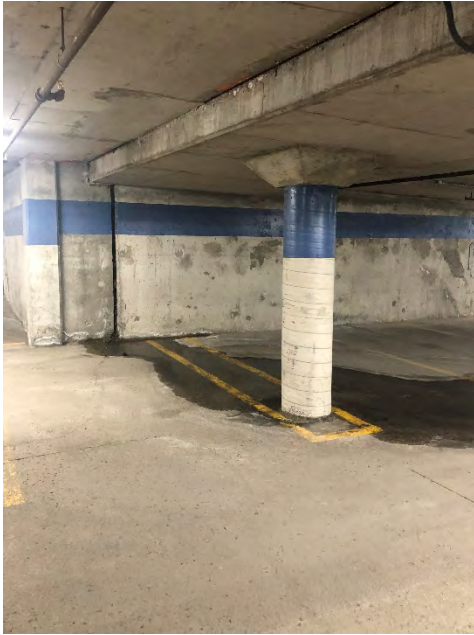
Photo 17 – Second sub-level parking, water leaking and pooling from a separation in the wall, looking east
