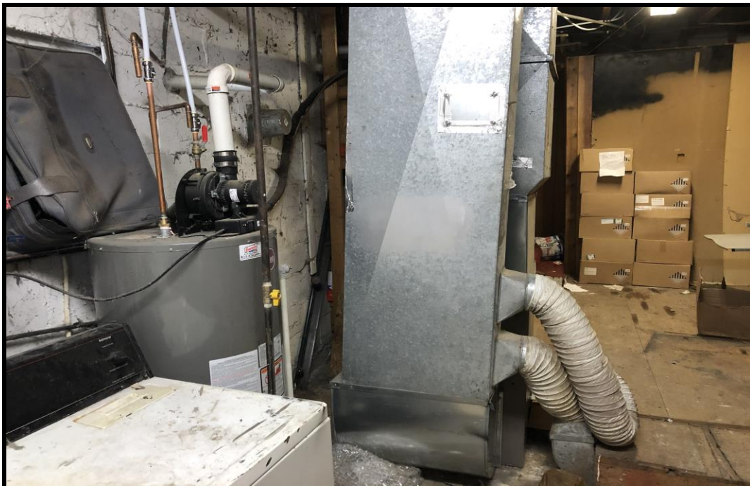
Photograph 4: View of the interior natural gas-fired furnace, located in the basement.
