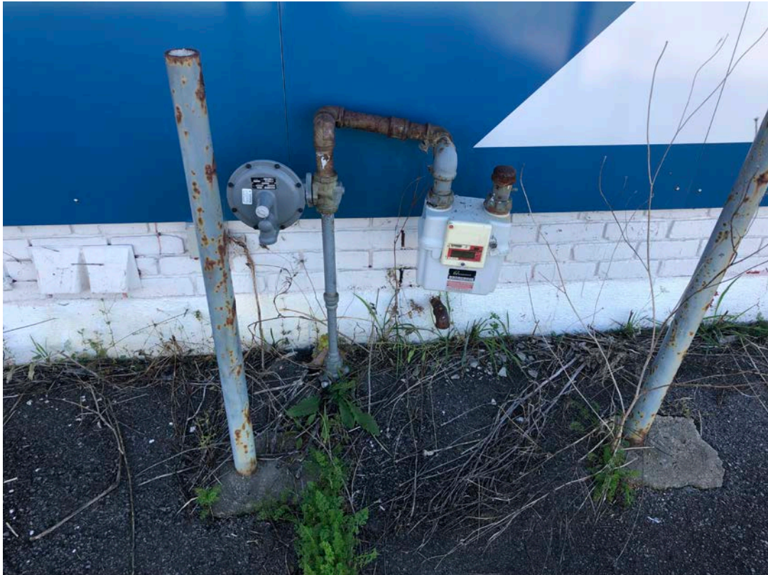
View of natural gas meter located along north side of building at the site
