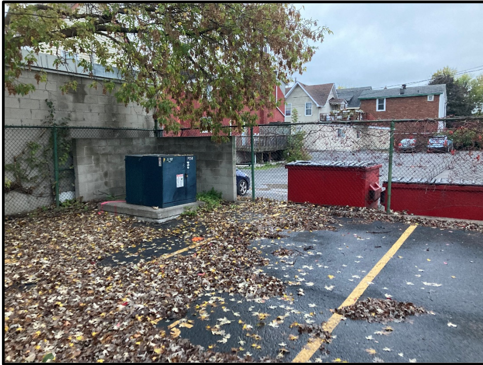
Photograph 5: View of the transformer located on the Phase I Property, looking south from within the Phase I Property.
