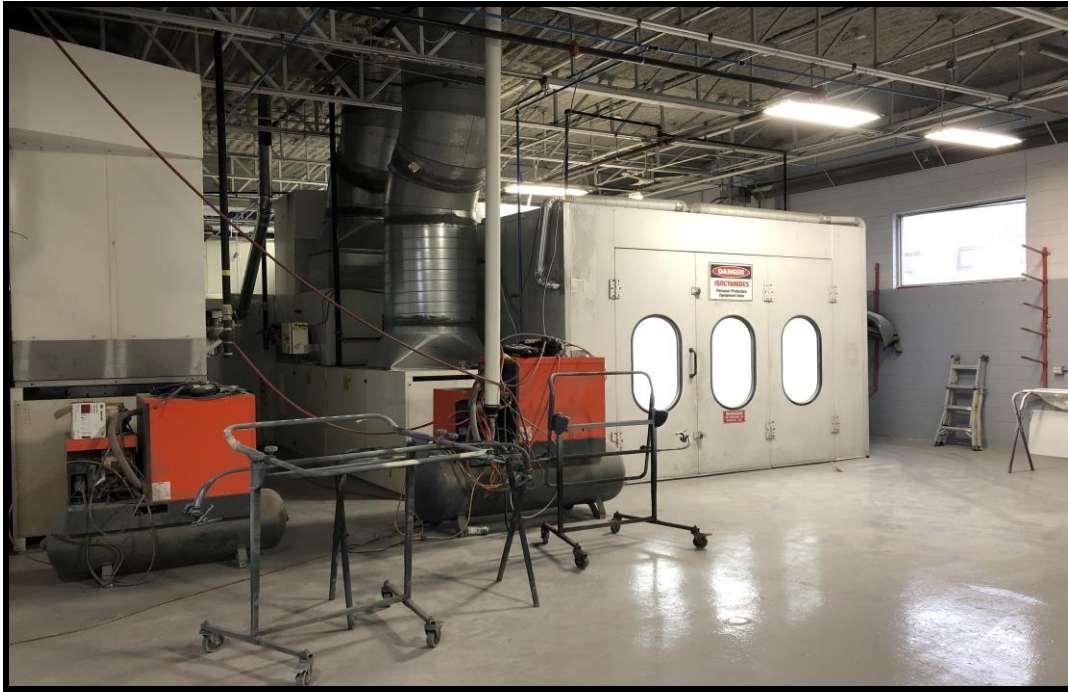
Photograph 5: View of an auto paint application booth, located inside of 40 Jamie Avenue.
