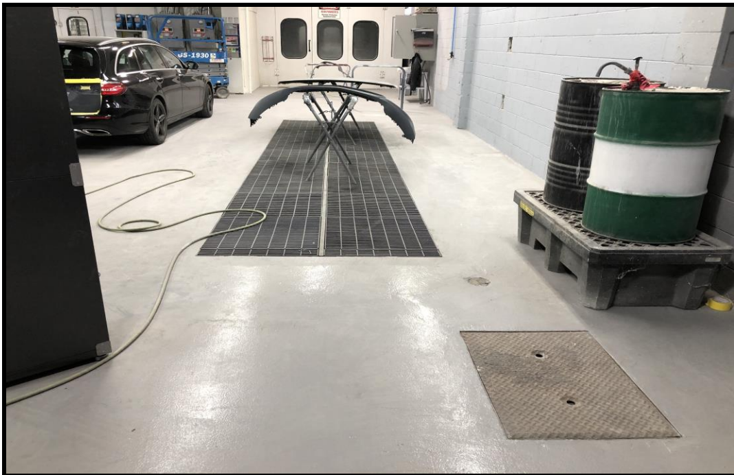
Photograph 6: View of a floor drain and water separator, located inside of 40 Jamie Avenue.
