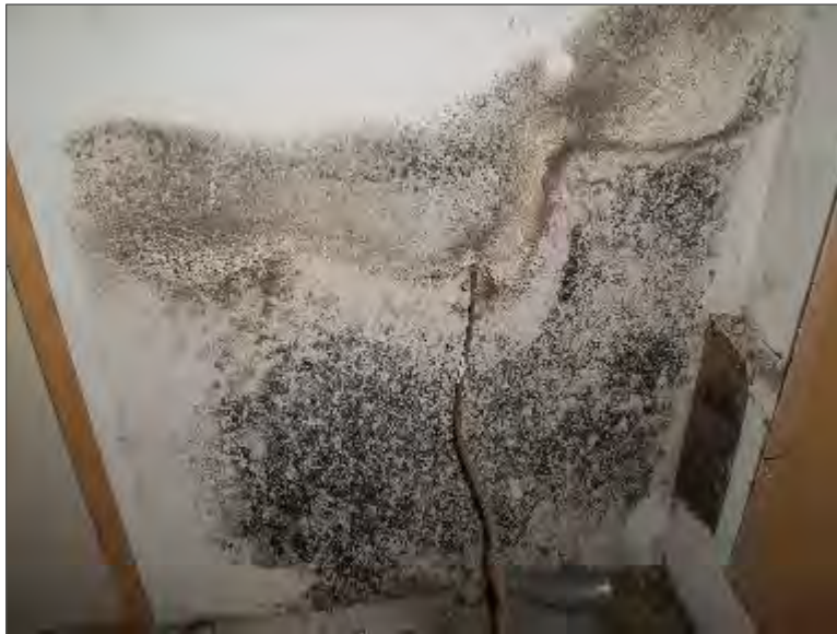
Photo 10 – Suspect mould growth observed on a gypsum board interior wall in the northeast portion of the Site Building.
