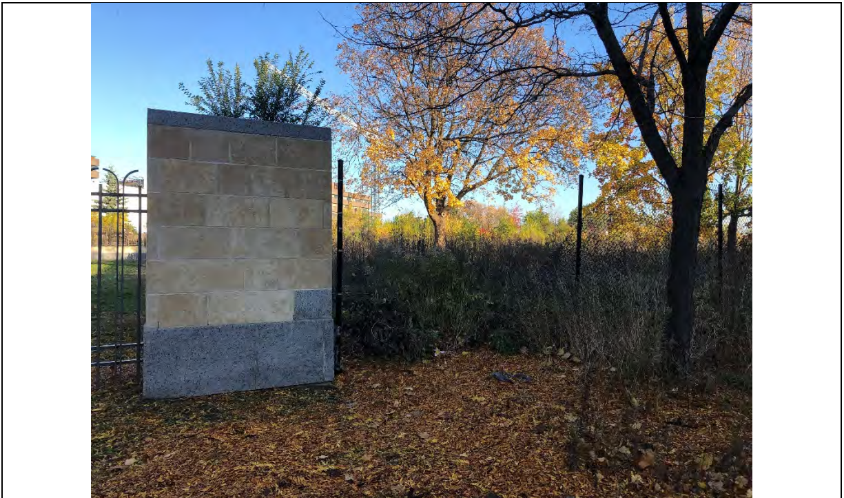
Photo 004 Damaged fence at the southwestern corner of the Phase One Property, facing north
