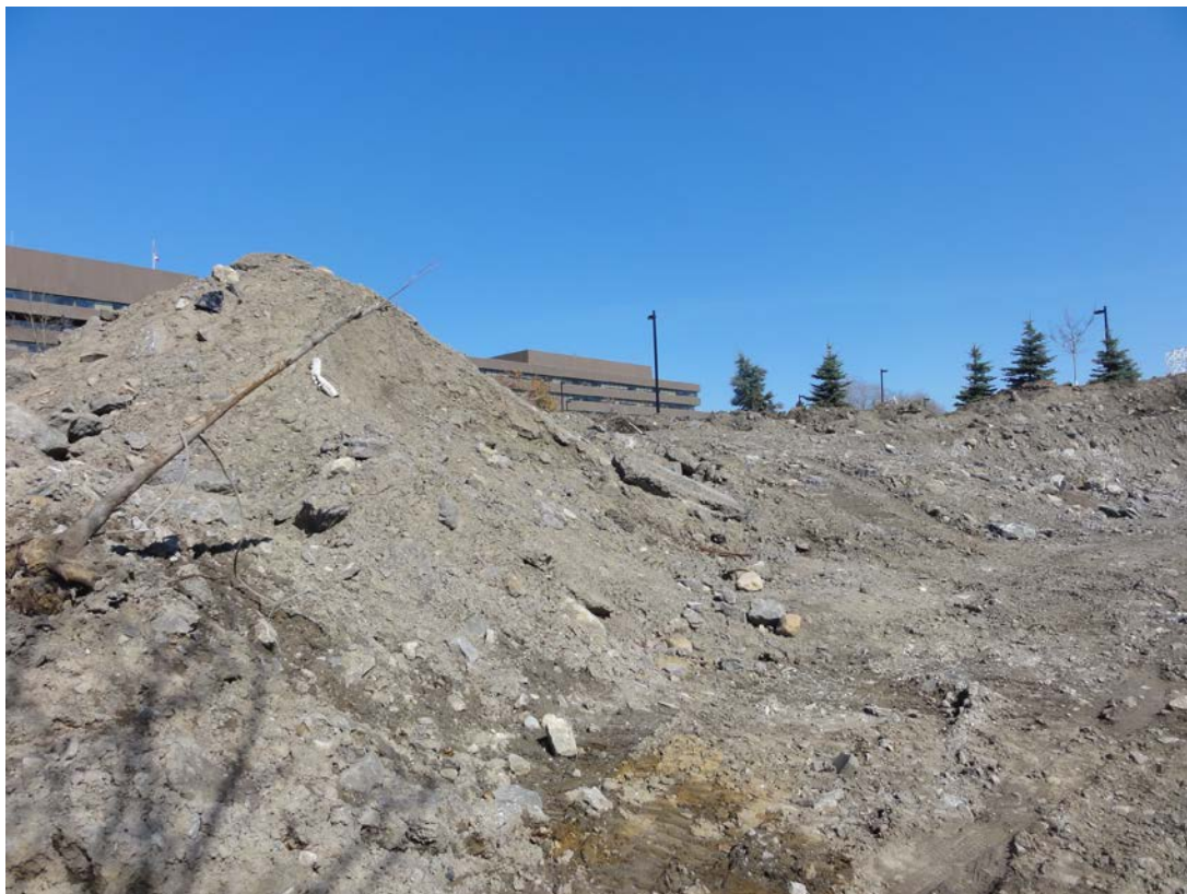
Photo 4: Soil berm present along the northern property line. 125 Sussex Avenue is visible in the background (April 22, 2013).
