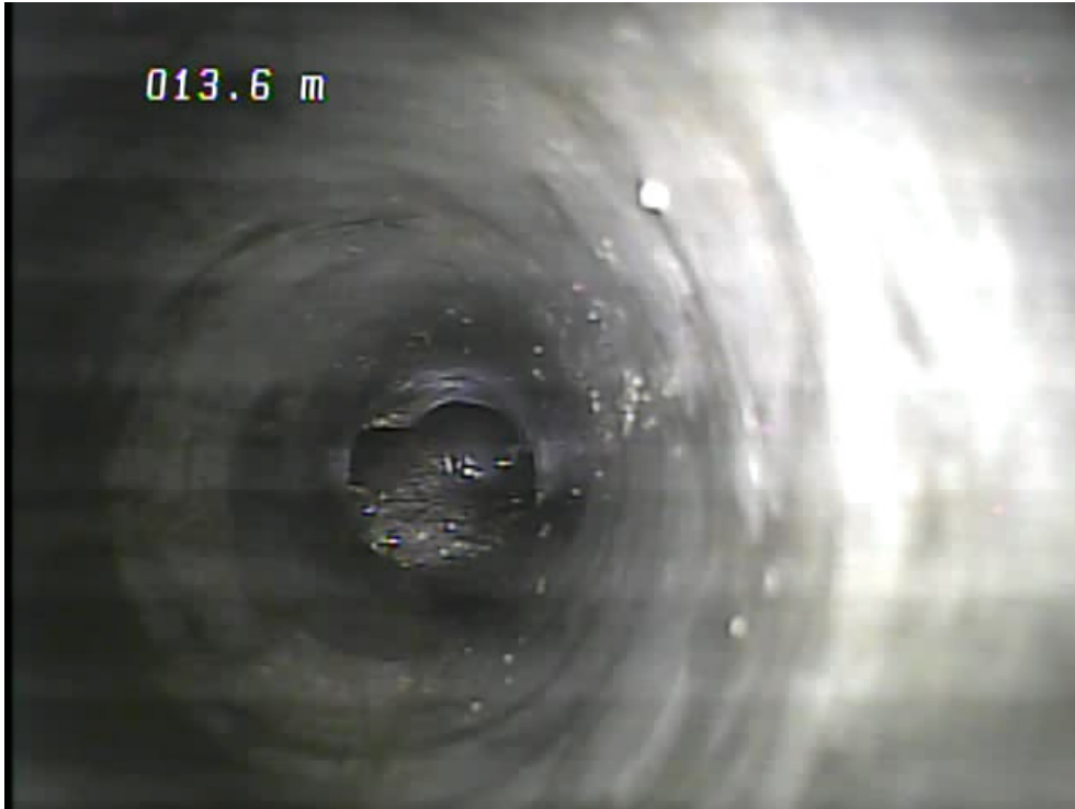
Photo 1: View down MW14-1, depth 13.2 m BGS, just above karst feature, visible in centre of photo.
