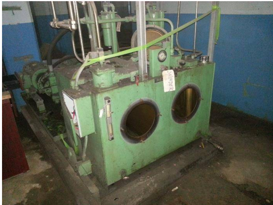
Photograph 8: View of lubricant oil AST in Building 503 basement, facing west (April 7, 2014)
