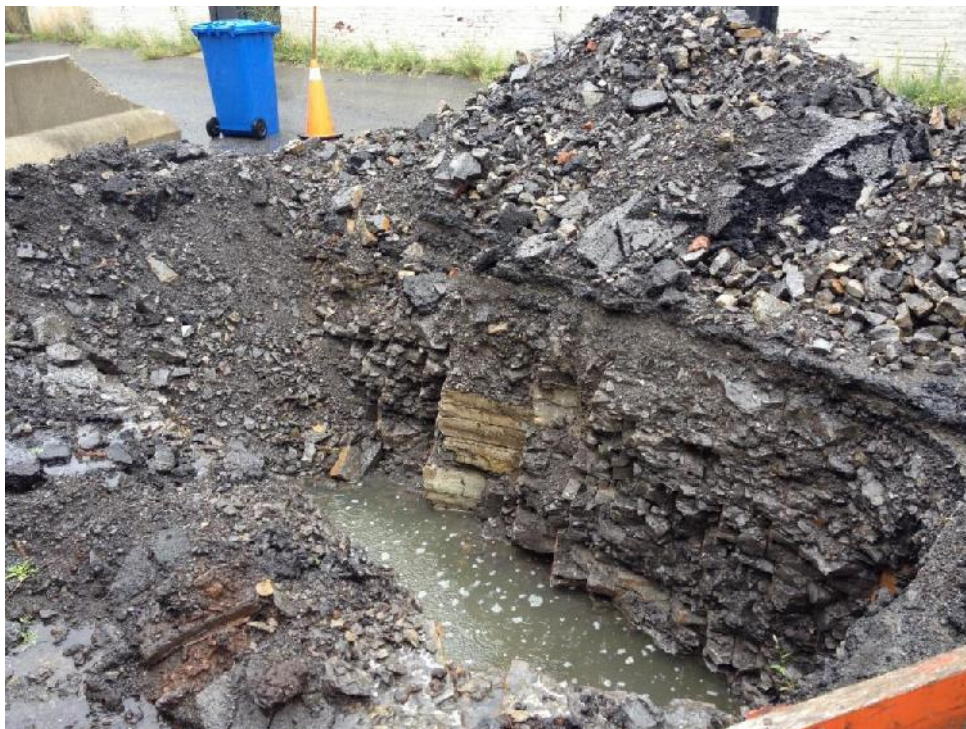
Photograph 16: Fill and shallow bedrock observed in an excavation on Albert Island (August 12, 2014).
