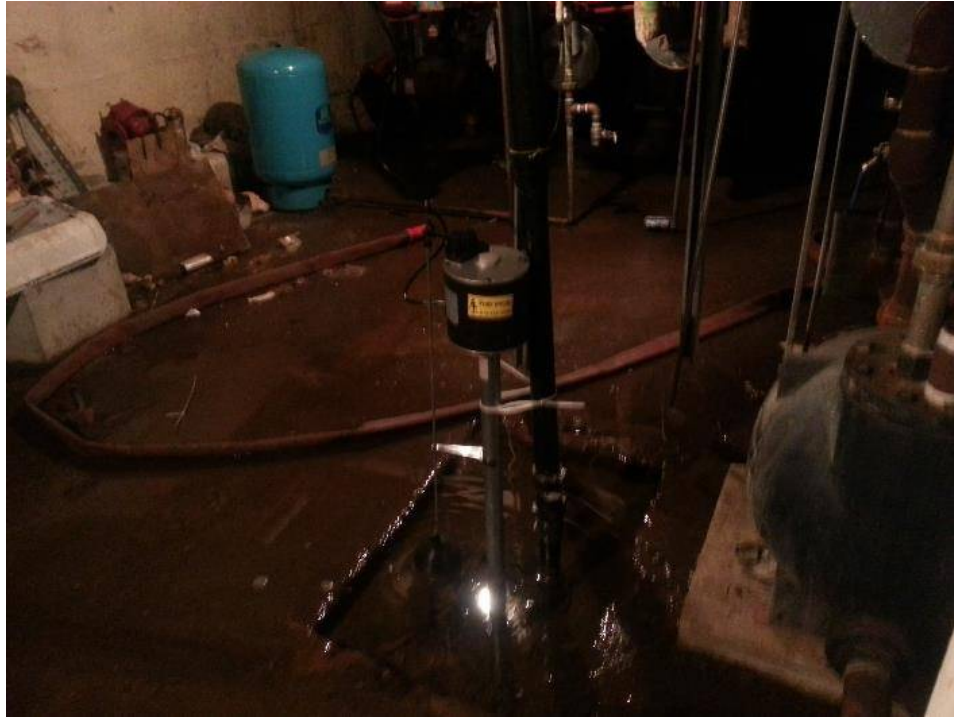
Photograph 9: View of sump pump in Building 541 basement, facing east (April 7, 2014)
