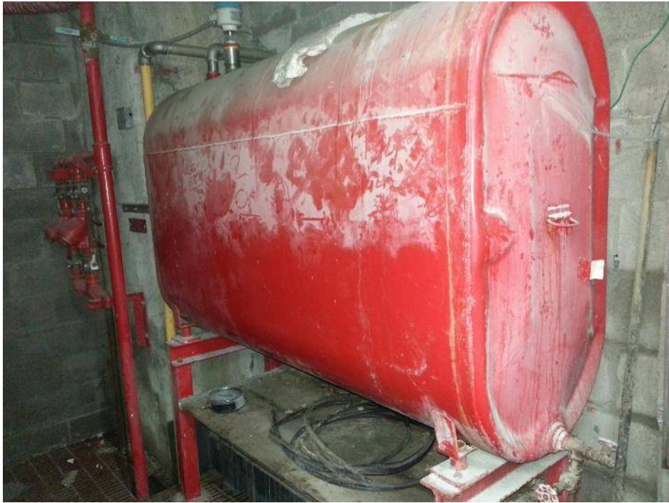
Photograph 7: View of diesel AST in Building 502 basement, facing south (April 7, 2014)
