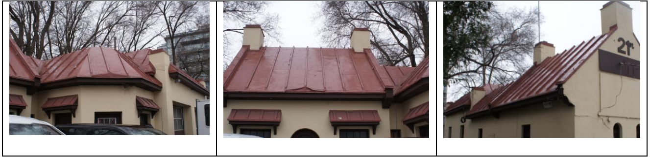
Figure 10: images of the standing seam roofs. Note the diverter flashing treatment above the doors.
