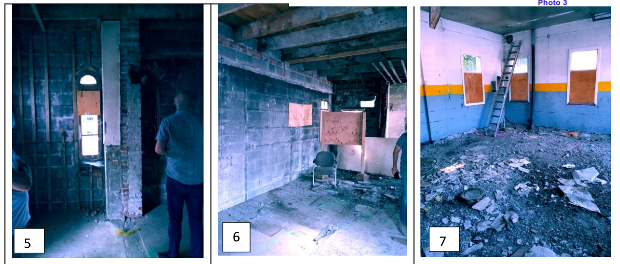
Figure 19: Interior views; 5. Looking towards the east wall with round headed windows on either side of the chimney. View 6. And 7. Interior views of transition area and the service bays. Source Commonwealth 2021
