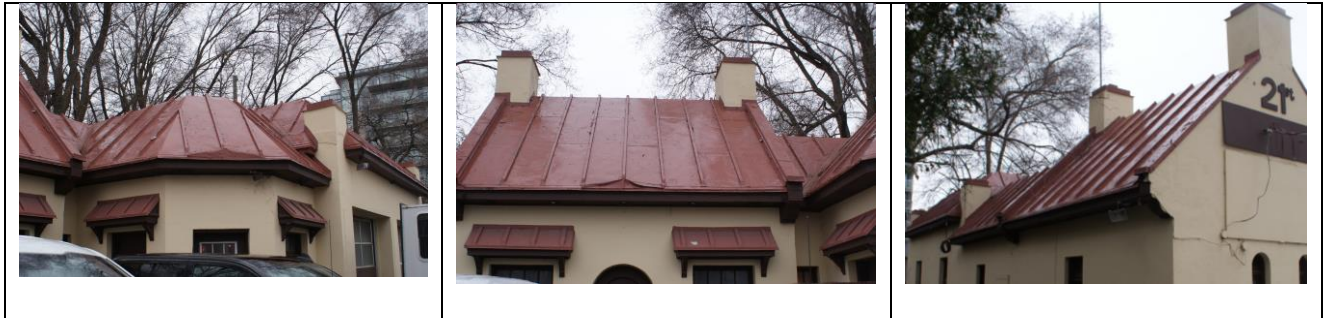
Figure 12: images of the standing seam roofs. Note the diverter flashing treatment above the doors.
