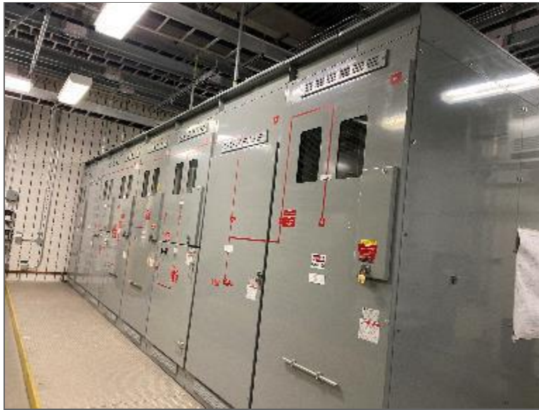
Photo 11 – Pad-mounted oil-cooled high voltage transformer (T1) located in the northeast portion of Site Building B (PCA/APEC).
