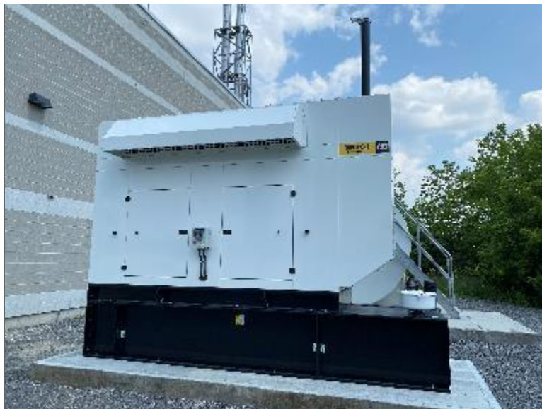
Photo 6 – 1,544-L belly tank steel AST, associated with an emergency generator, located exterior to the southwest elevation of Site Building B (PCA/APEC).
