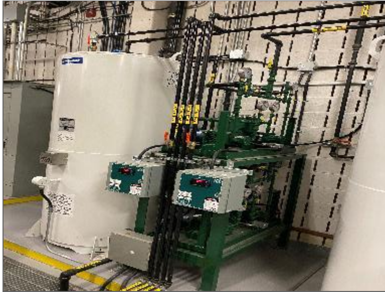
Photo 9 – 1,663-L double-walled steel AST containing diesel located in the central portion of Site Building B (PCA/APEC).
