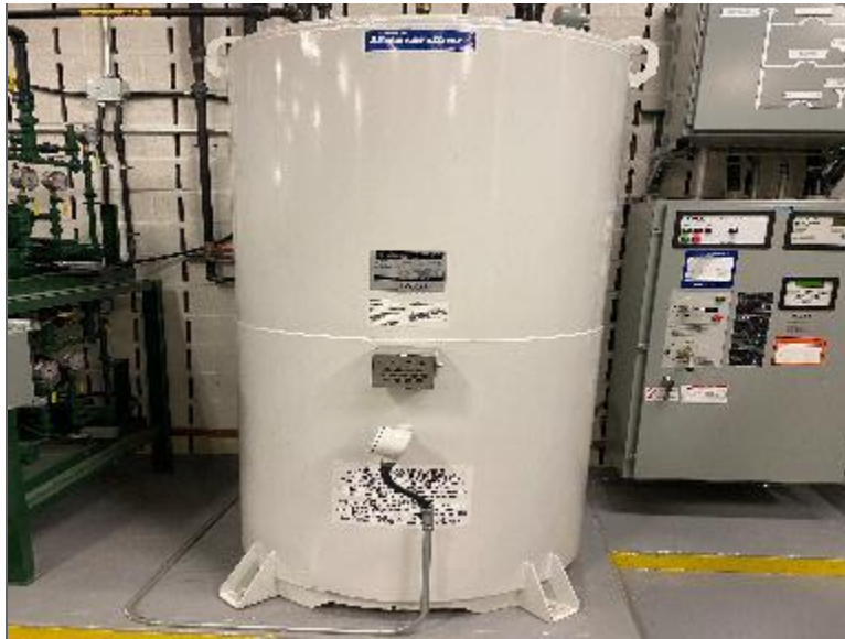
Photo 10 – 1,663-L double-walled steel AST containing diesel located in the southeast portion of Site Building B (PCA/APEC).
