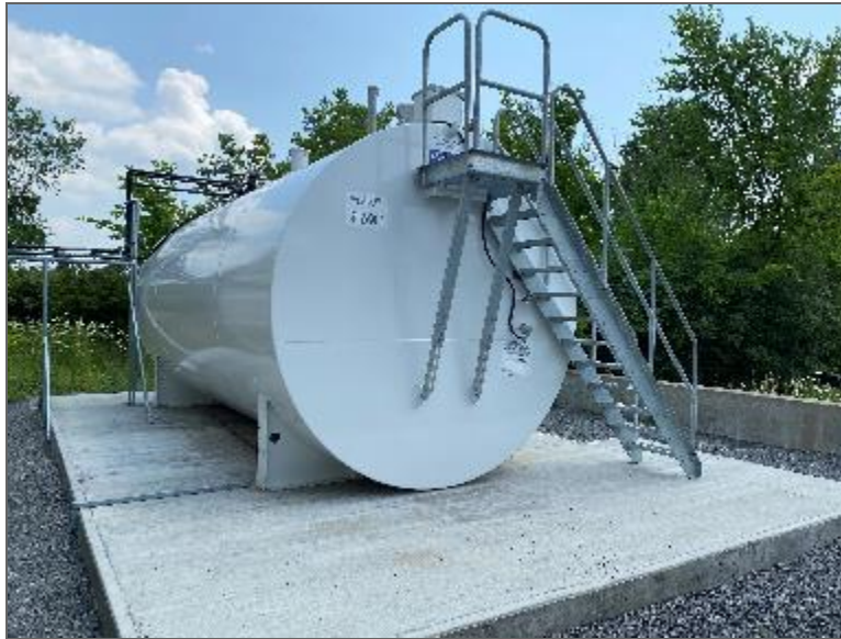
Photo 5 – 45,698-L double-walled steel AST located exterior to the southwest elevation of Site Building B (PCA/APEC).
