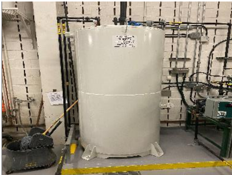
Photo 8 – 1,663-L double-walled steel AST containing diesel located in the northwest portion of Site Building B (PCA/APEC).
