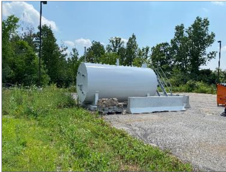
Photo 7 – 24,974-L steel AST, reportedly empty and not in use, located exterior to the southwest elevation of Site Building B (PCA/APEC).
