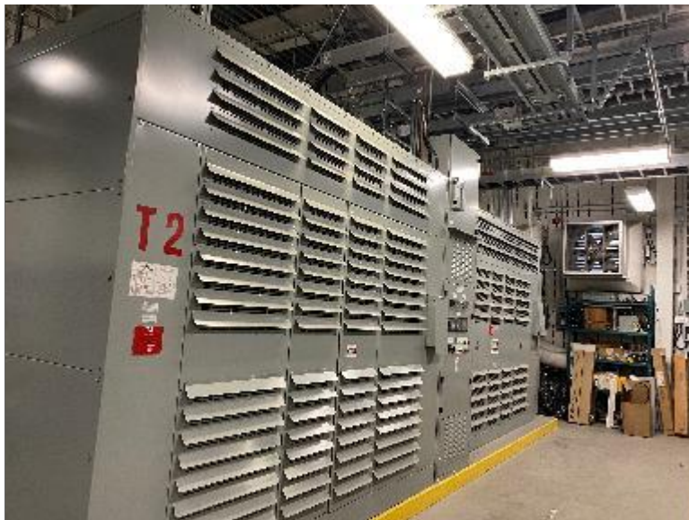
Photo 12 – Pad-mounted oil-cooled high voltage transformer (T2) located in the northeast portion of Site Building B (PCA/APEC).
