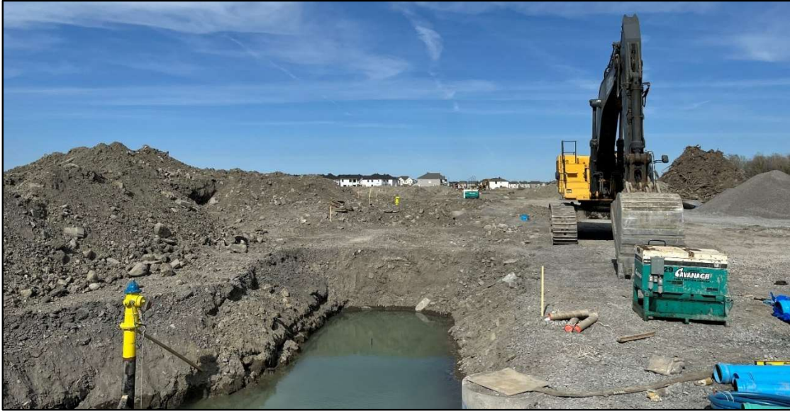
Exhibit E: Photograph facing east along the future extension of Flagstaff Drive, with the Subject Property to the right of the open servicing trench.
