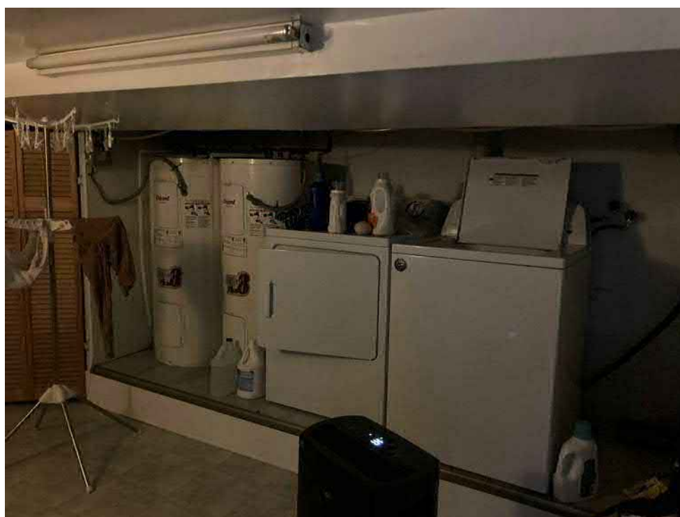
Photo 4: View of the laundry room in the basement of the building.
