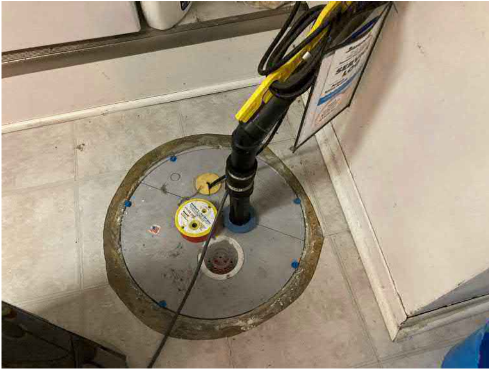
Photo 5: View of the sump pump located in the laundry room of the basement.
