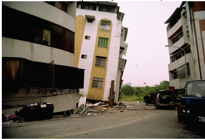
(b) 5- and 6-story buildings with foundation failures near the locations of borings WAS-3 and WAS-4 (photo by R. B. Seed)
