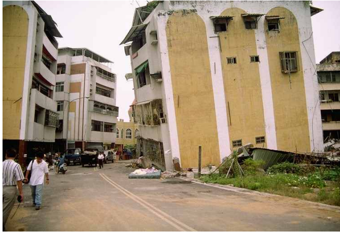
(a) 5- and 6-story buildings with foundation failures near the locations of borings WAS-3 and WAS-4 (photo by R. B. Seed)
